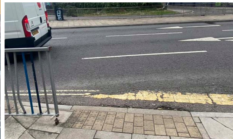
Tactiles indicate crossing where no crossing exists
